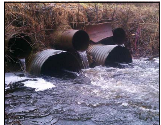
Figure 2. The culvert system at E Drive on Pigeon Creek, a tributary of the Kalamazoo River, prior to restoration of fish passage.
